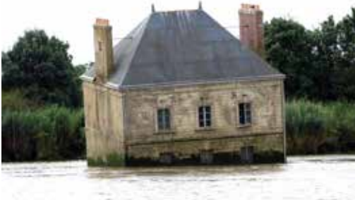
Gentleman's residence on the River Loire with a slight damp problem
