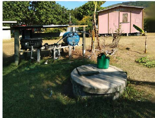
A completed solar desalination unit ready to start work
